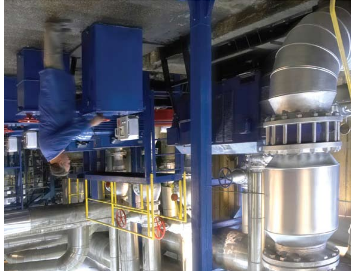
> Pump and HVAC
